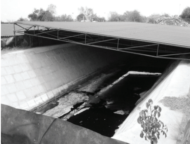
Liquid waste stored in concrete underground tank
